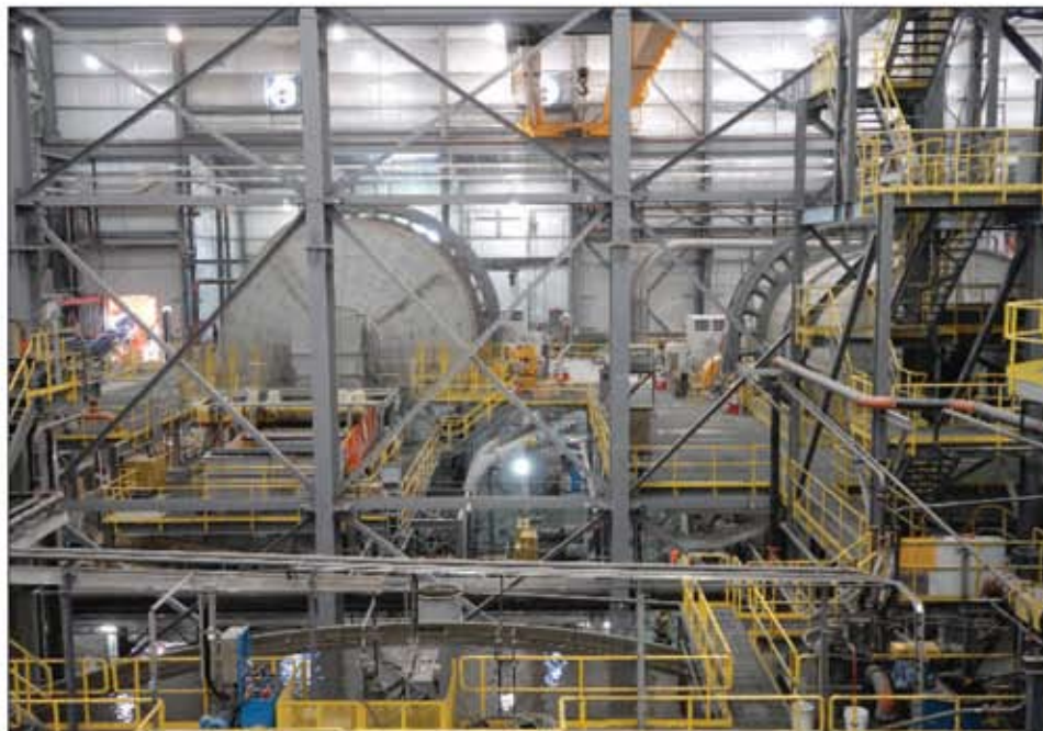
An interior view of the new process plant at Copper Mountain. The SAG (semi-autogenous grinding) mill is pictured on the left, ball mill on the right and concentrator thickener in the foreground. Photos courtesy Copper Mountain Mining Corporation.
